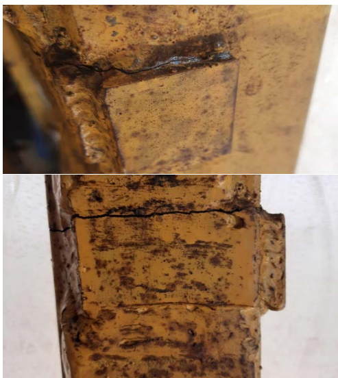
Fig. 2. Damage in the form of cracks in the head of the LIEBHERR 185HC tower crane in Kyiv
